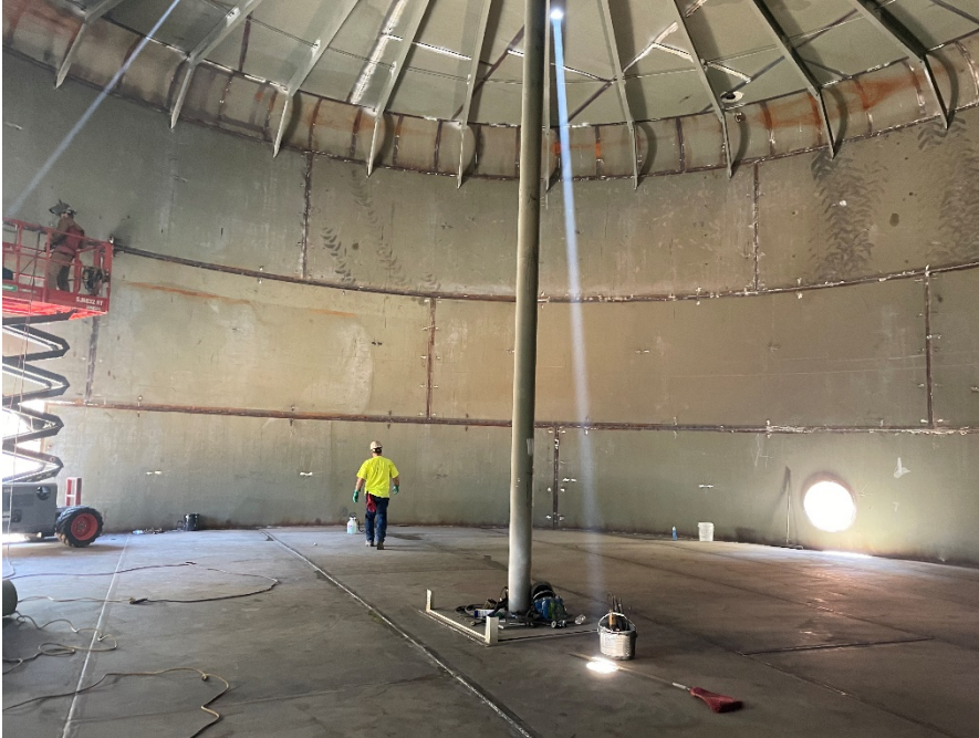
Interior of Tank 2 prior to coating – green color is the zinc primer
